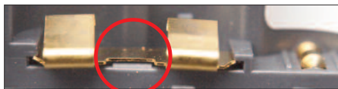
Photo 13: Battery contact not properly locked in position
